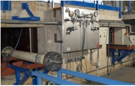
Airborne's in-house pressure test facility
